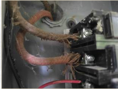
Cloth sheathed wiring method present, an upgrade is highly recommended
