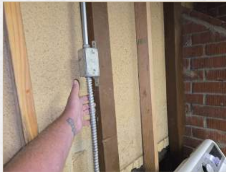
Unsecured or loose wiring/conduit/electrical, recommend repair or replace
