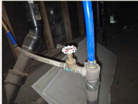
Polybutylene plastic plumbing present, we recommend a complete water distribution system evaluation in areas
