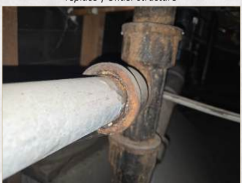
Cast-iron drain pipes rusted/corroded, recommend repair or replace
