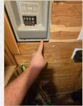
Missing screws at closet
