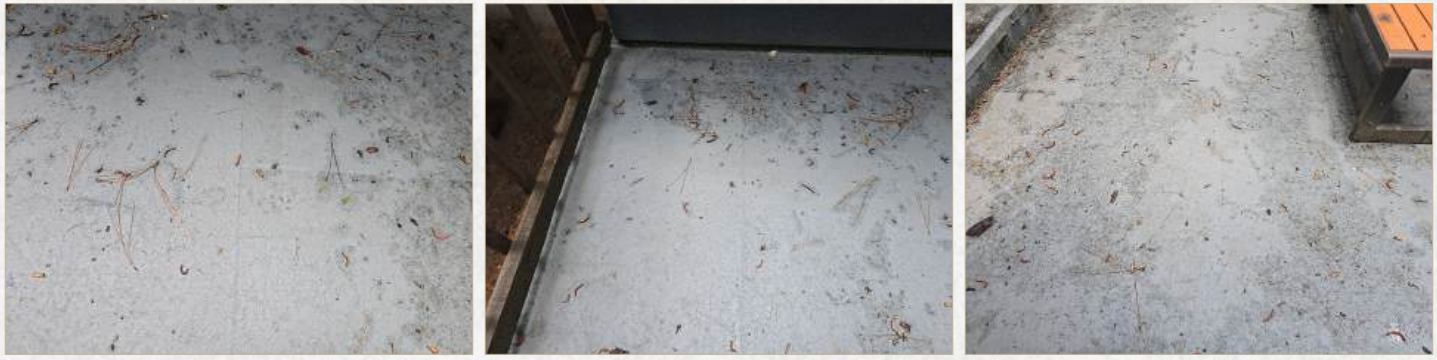
Cracking/exposed seams, recommend maintenance
