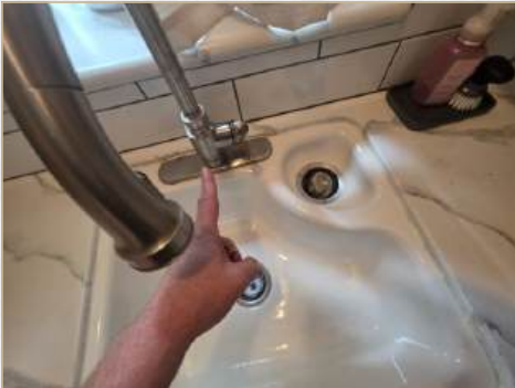
Loose fixture/handles, recommend repair or replace
