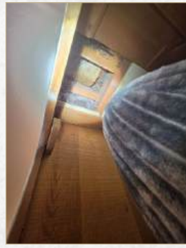
Stains/unfinished area(s), tested dry at time of inspection, monitor area for moisture | South bedroom
