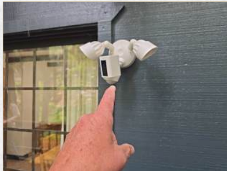
Fixture did not operate, recommend repair or replace | East side of structure
