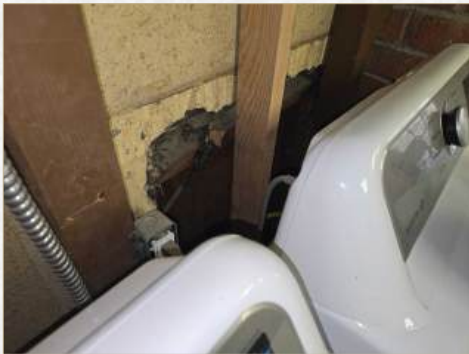
Holes present in fire wall, recommend repair or replace to retain integrity of fire separation
