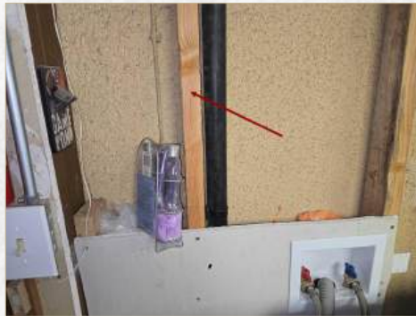
Missing fire rated materials, recommend repair or replace to retain integrity of fire separation
