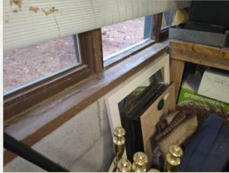
Stains/blisters at sill, tested dry for moisture at the time of the inspection, monitor the areas for moisture intrusion
