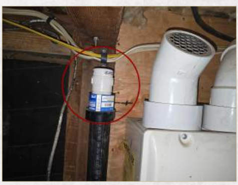
Air admittance valve present, recommend repair or replace | Under structure
