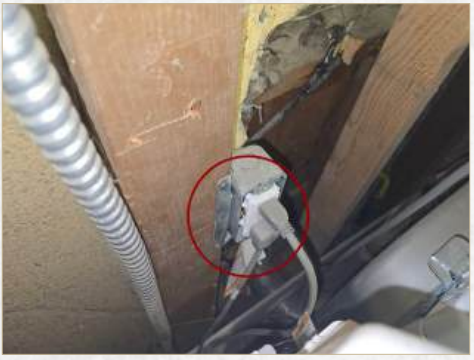
Laundry outlet(s) have been upgraded with no GFCI protection (upgrades must meet new electrical requirements), recommend further evaluation
