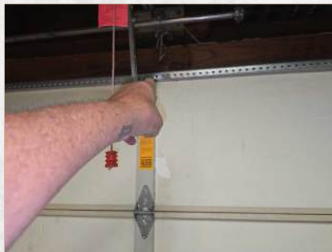
Cracked in areas, recommend repair or replace
