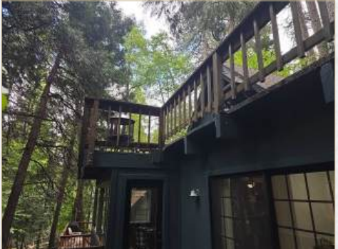
Handrail/guardrail openings too wide, normal for age, 4" maximum recommended for safety
