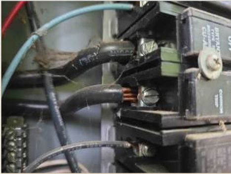
Wire insulation over-stripped exposing too much bare wire, recommend further evaluation
