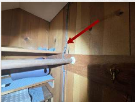
Nonmetallic cable (NM)/Romex wiring exposed, recommend repair or replace | 2nd floor North bedroom
