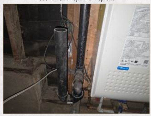
Open vent, recommend repair or replace | Under structure
