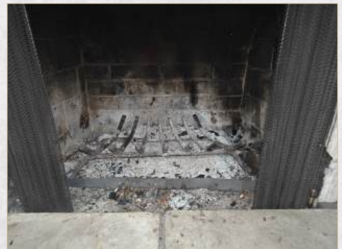
Fireplace dirty, recommend cleaning by a CSIA chimney inspector/sweep
