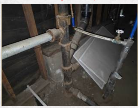
Cast-iron drain pipes rusted/corroded, recommend repair or replace
