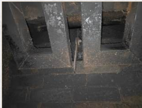
No damper stop clamp, required for cosmetic gas logs, fire-glass or other cosmetic fire system that uses gas at the primary fuel
