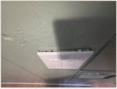
Loose outlets, recommend repair or replace | Game room
