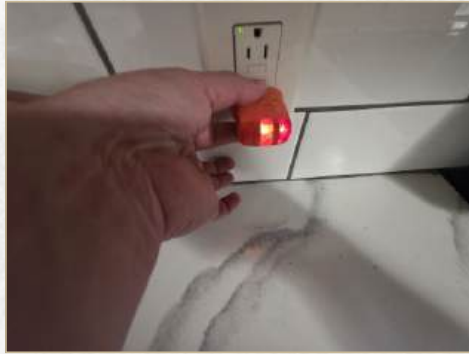
GFCI not grounded, typical for old Ungrounded system pre-1965
