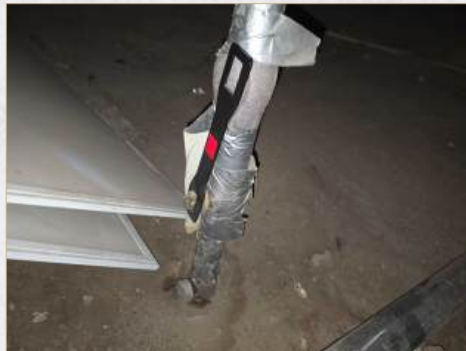
Improper shut off valve, using gas valve for shut off, recommend repair or replace
