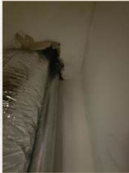
Large holes or cracks observed, recommend repair or replace | Closet/Cabinet
