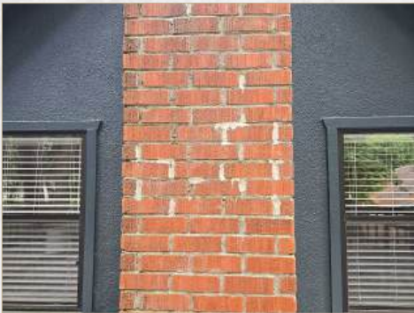
Step cracking present, recommend repair or replace
